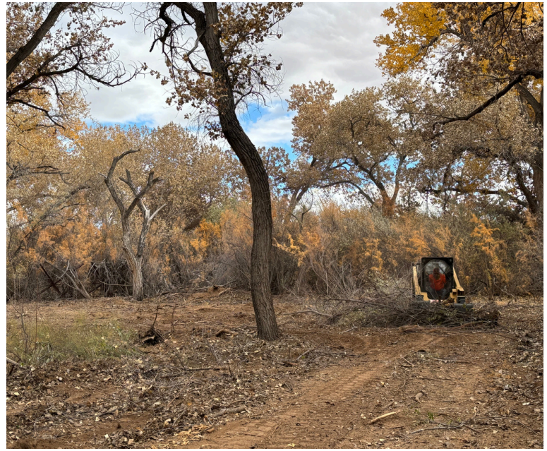
Forestry contractor use heavy machinery to extract salt cedar, reducing the use of herbicide. Restoration to native, more water conscious vegetation will begin when area has been cleared out.
