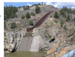
Photograph shows spillway, outlet works and the stilling basin in the foreground, taken fall of 1995
