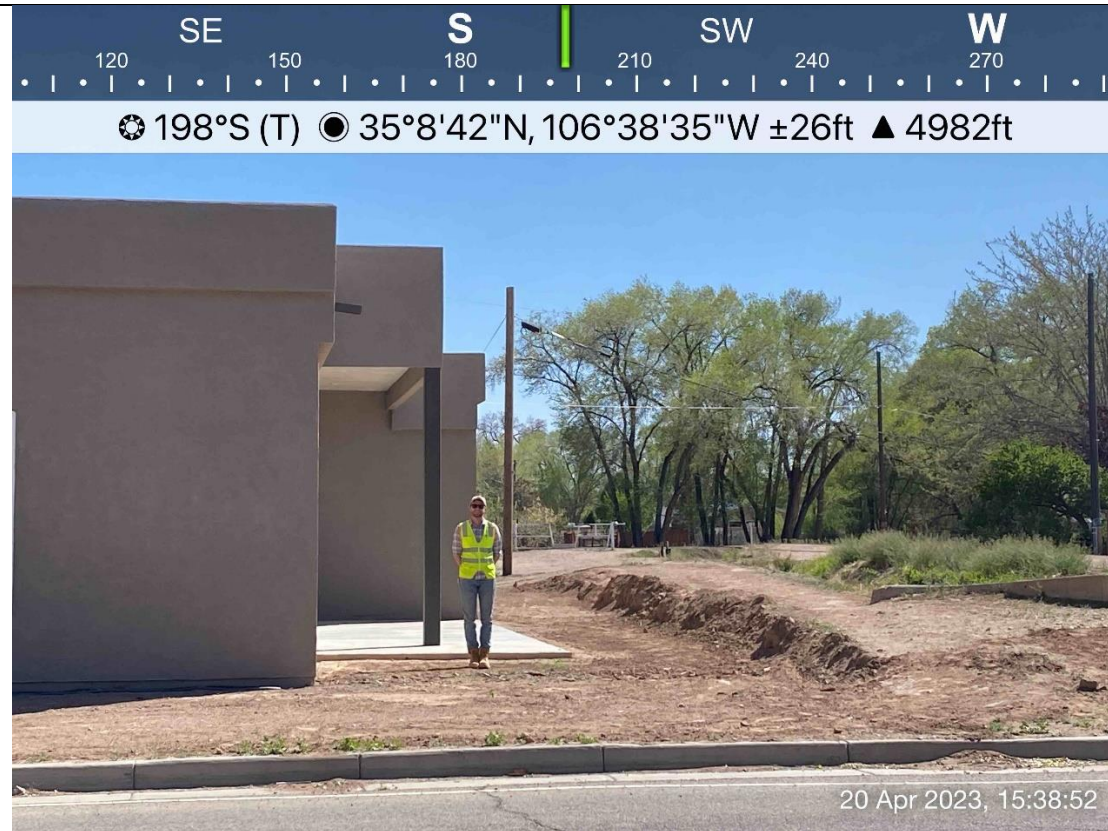
Photo 1. View of cut into eastern maintenance bank of Harwood Lateral from Tract 16C, looking south from Grecian Ave NW. Note the narrow distance between the concrete wingwall for the outlet structure and the new outer edge of the bank.
