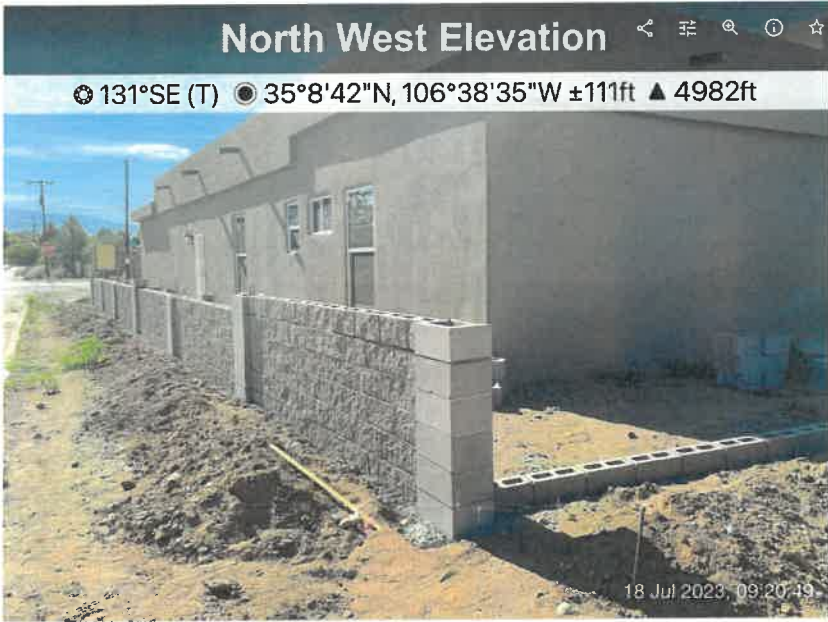
Figure C. Extent of block wall constructed as of July 18, 2023, showing portion of wall to be constructed along disputed boundary of MRGCD right-of-way and private property.
