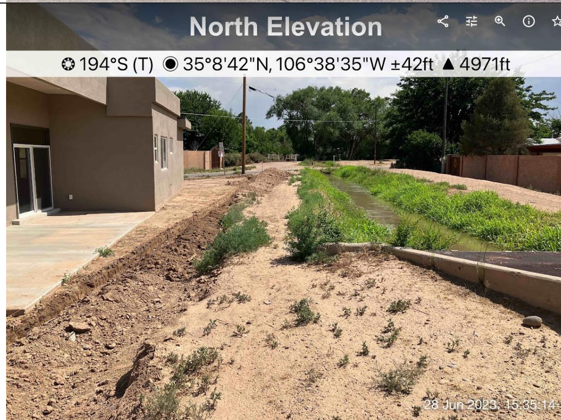
Photo 2. View of footing for block wall dug in late June, looking south from Grecian Ave NW.
