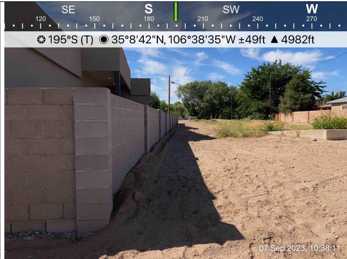
Photo 5. View of completed wall. Notice dirt returned to ditch bank resting high on wall.
