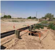
Isleta Interior Drain at Hwy 147, Sink Hole 2021
