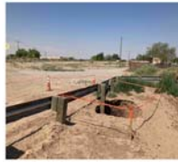
Ilieta Interior Drain at Hwy 147, Sink Hole 2021
