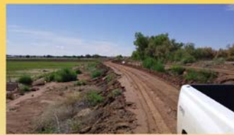
San Antonio Ditch Overtopping Damage
